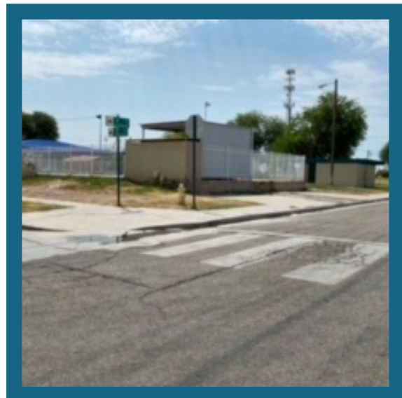
IMAGE: CROSSWALK WITH NO RAMP
