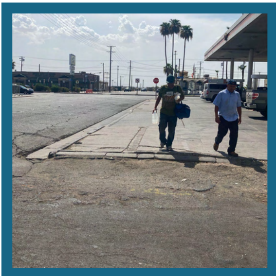
IMAGE: CRACKED SIDEWALK
