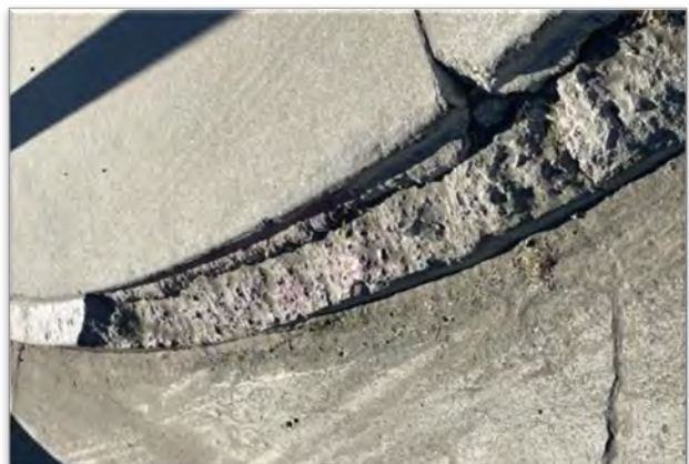
Broken Curb at Sandison/Drumm
