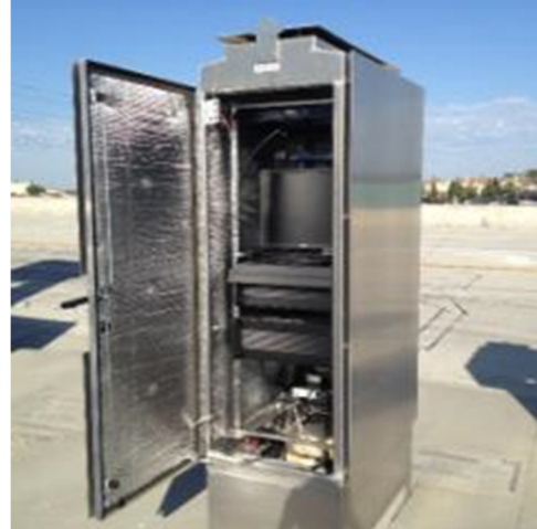
Figure 8-2: Lane Controller Cabinet
