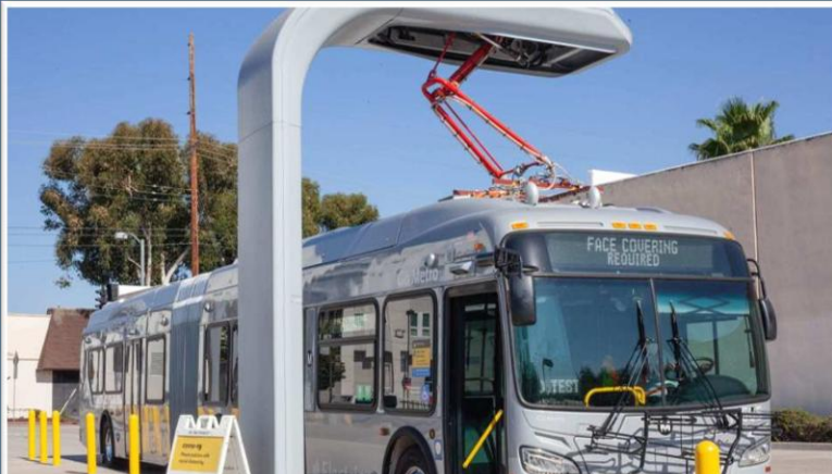
On-Route Overhead Charging
