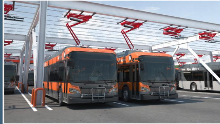
Depot Overhead Charging
