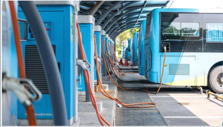
Depot Plug-in Charging
